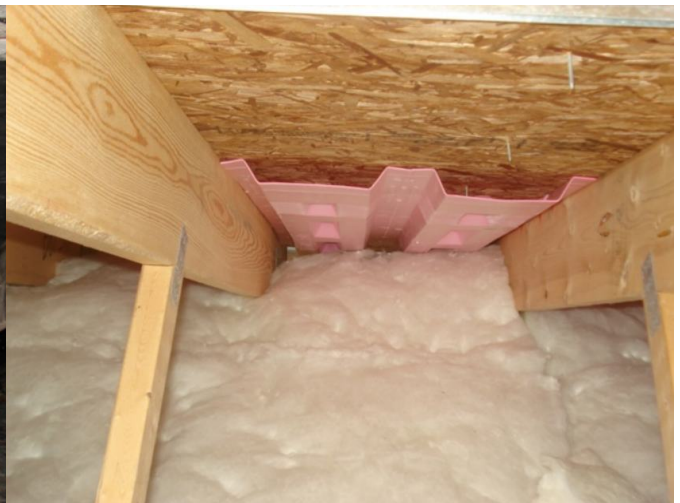
Properly Vented Attic
