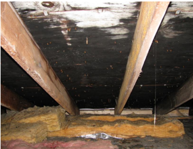
Mold growth inside un-vented attic
